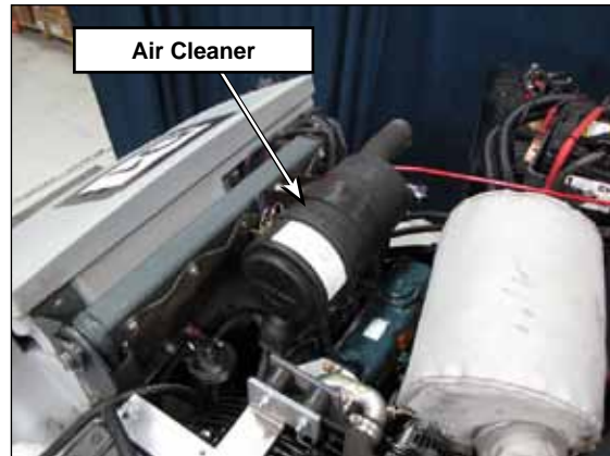
Top of engine compartment with top covers removed
