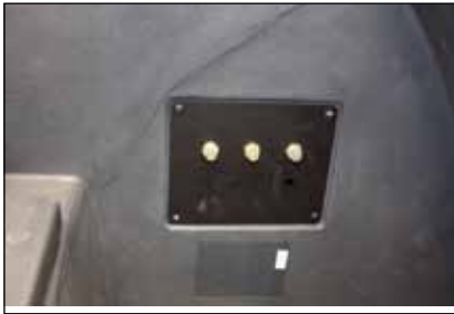
Circuit Breaker Panel
